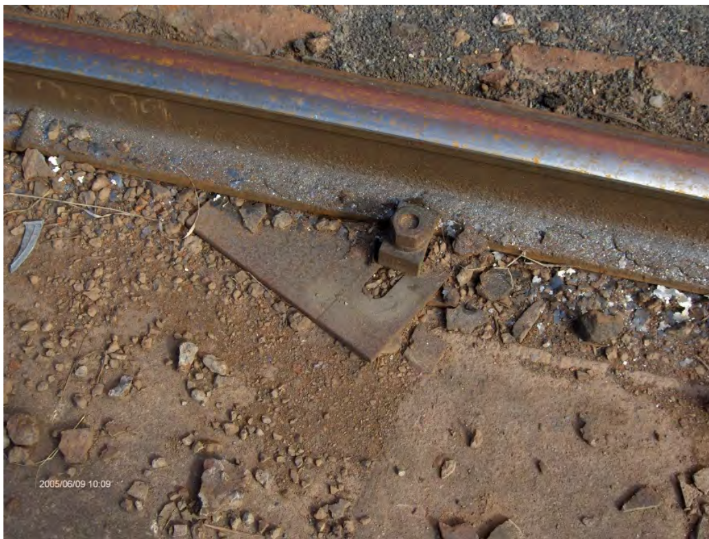
Figure 15: Damaged rail system
