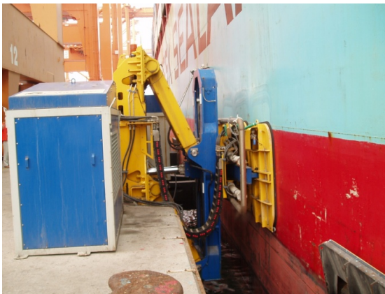
Figure 8: MoorMaster™ Unit on Container Berth
