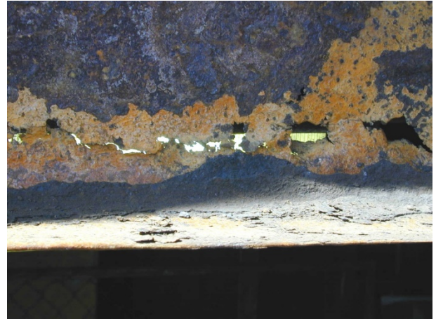
Figure 10: Corroded Steel Section
