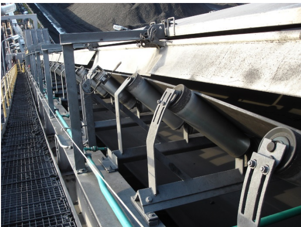
Figure 1 Conveyor idlers supporting a conveyor belt.
