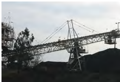
Radial Stacker Peak Downs Mine
