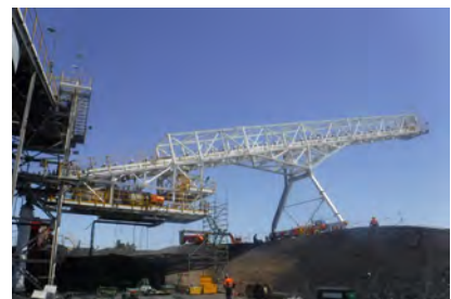
Radial Stacker BMA Blackwater Mine
