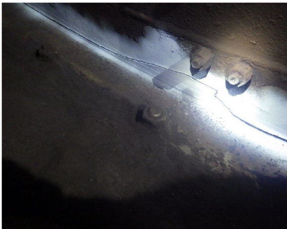
Figure 2 - FULT model damage ratio plot (top) showing areas on the car dumper end ring structure with low fatigue lives (red areas). The photo at bottom shows a circumferential crack running along the fillet of a rolled T-section in the car dumper end ring.
