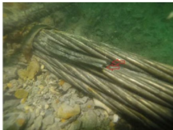
Figure 1 – Damage of prestressing wires in redundant approach caisson (Source: BMA)
