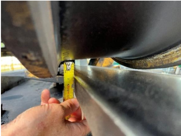
Figure 5 - Machine leg uplift at wheel level.
