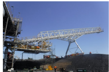
Radial Stacker BMA Blackwater Mine
